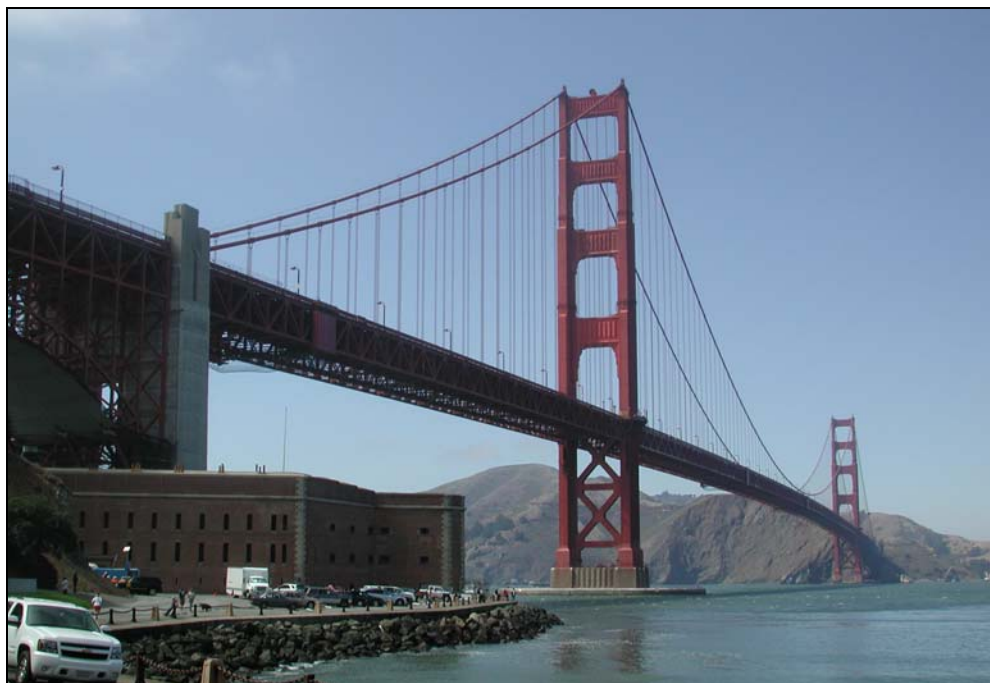
Photograph 2. View of east side of bridge from Fort Point, camera facing north, August 2007. [Source: MacDonald Architects]
